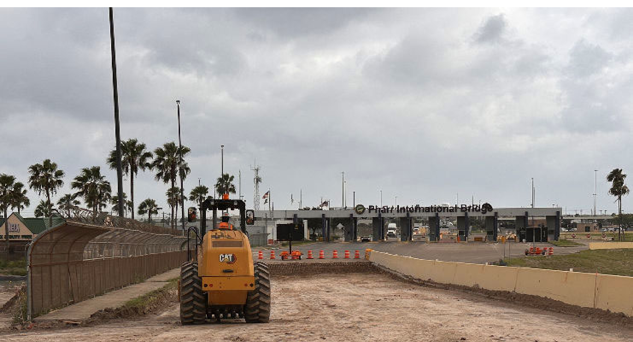
06-19-2026 – the contractor continued embankment operations by performing additional compaction throughout the lime-treated area.
