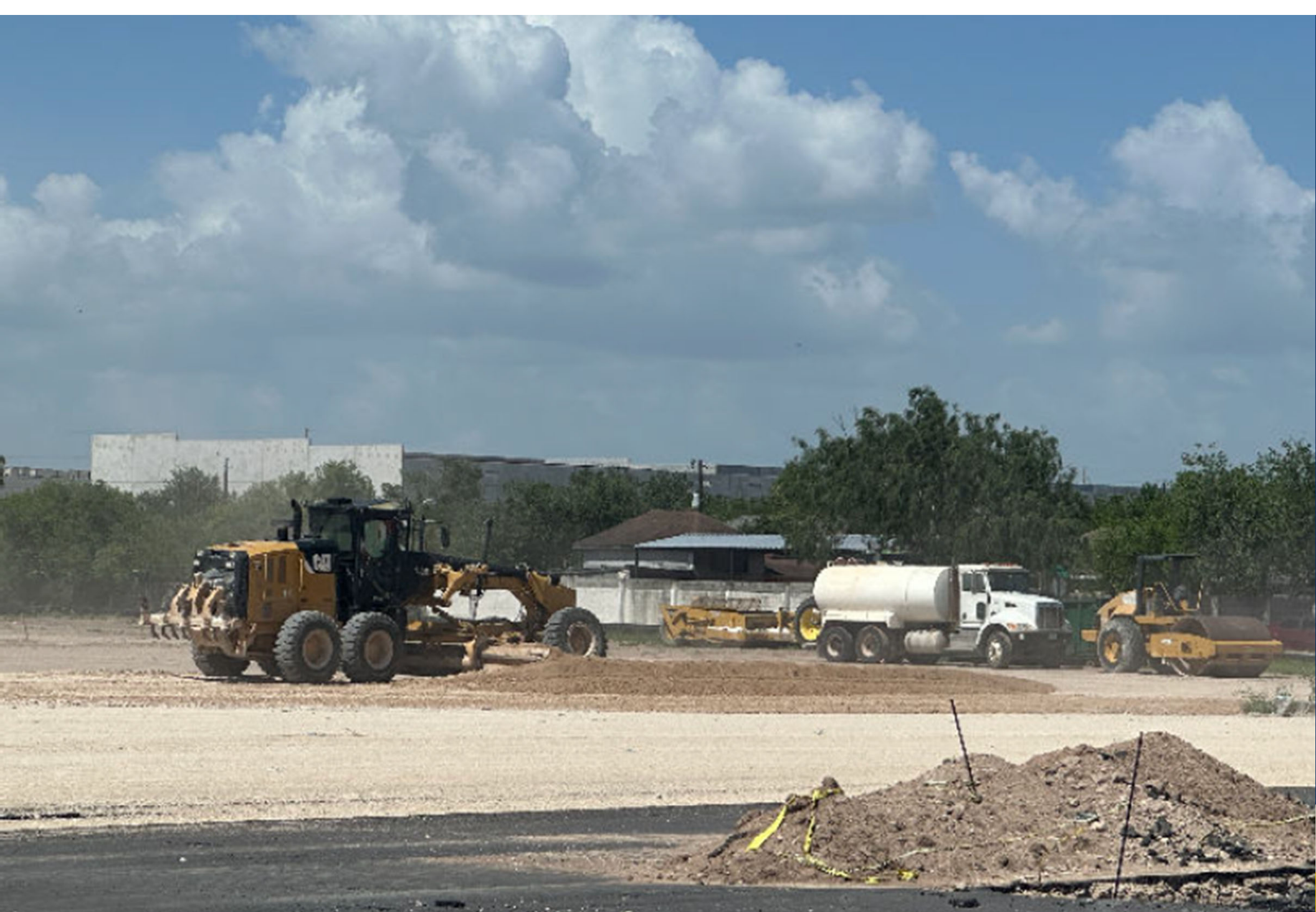
06-23-2026 – the contractor continued general house keeping and delivery and placement of new base material
