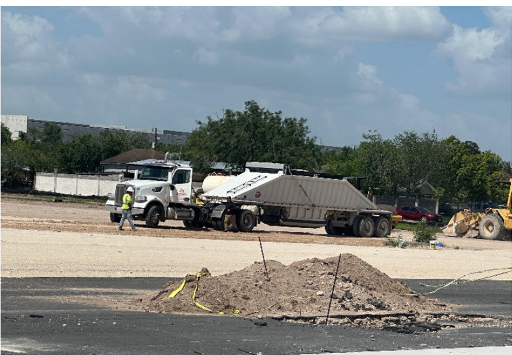
06-23-2026 – the contractor continued general house keeping and delivery and placement of new base material
