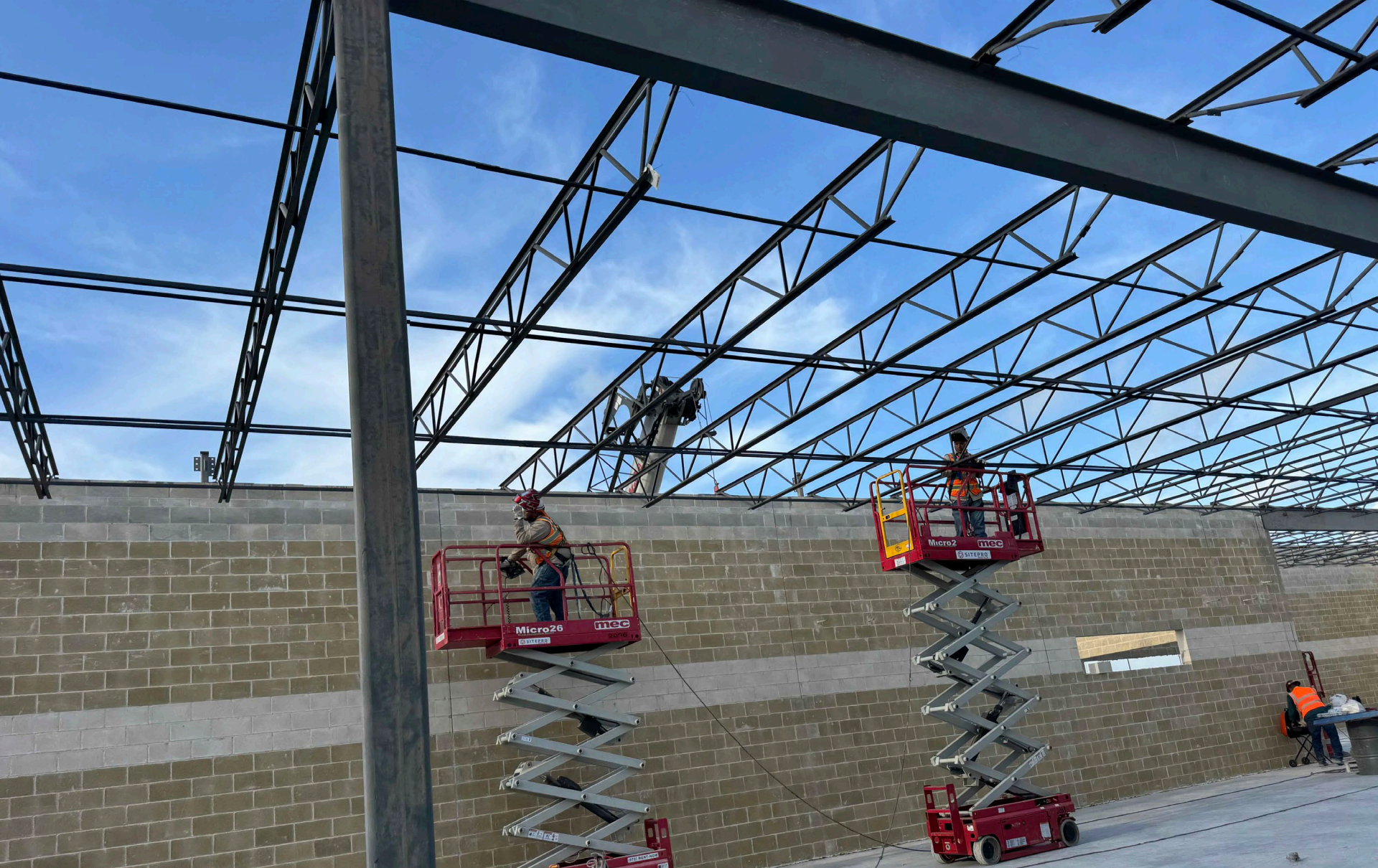
04-02-2026 – the contractor continued installing steel bridging for the steel joist in the Agricultural Building.
