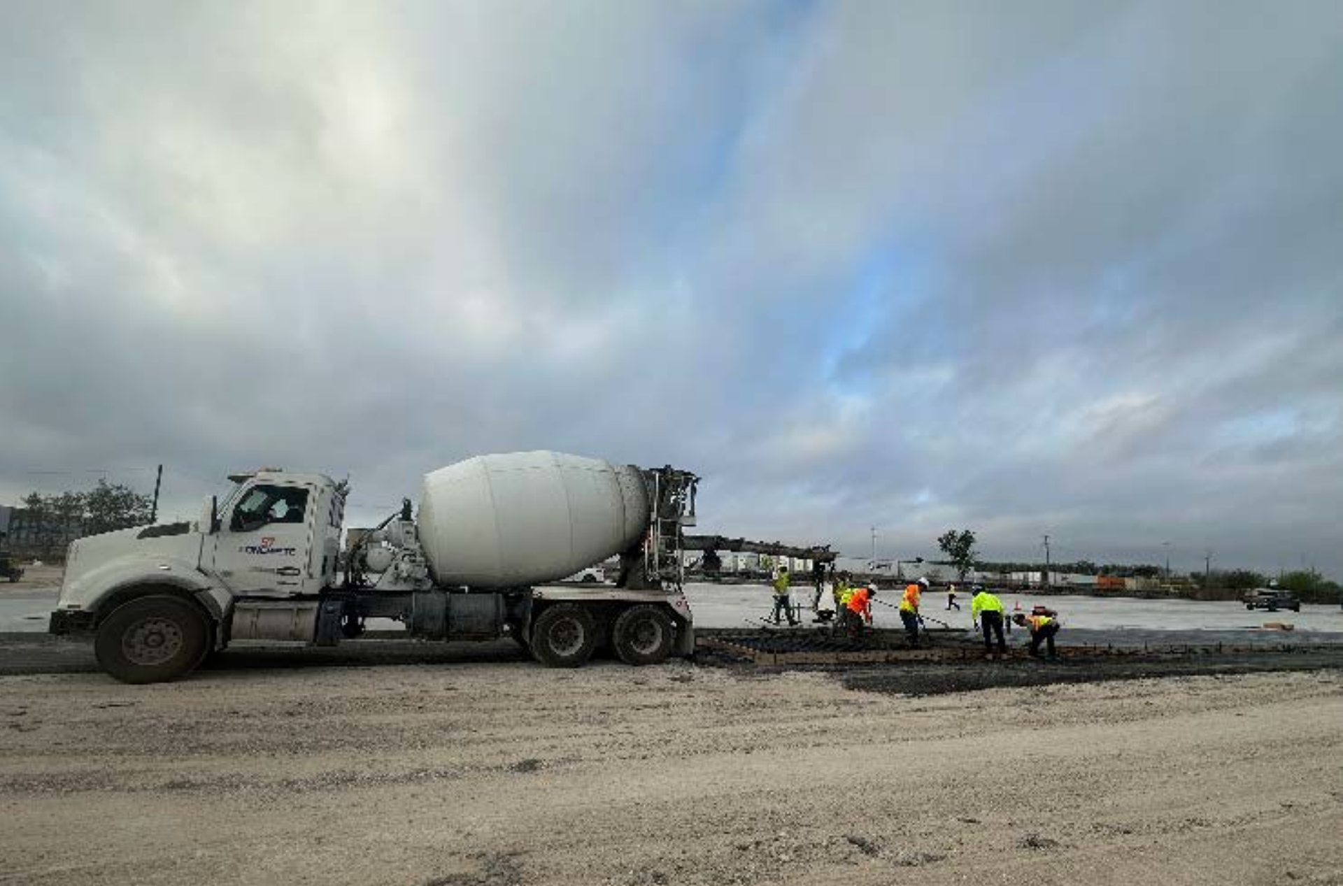
03-05-2026 – The Maverick Company crew placed 7.5-inch Continuous Reinforced Concrete Pavement in Sections 3 and 4. Operations included concrete delivery, placement, consolidation, finishing, and general housekeeping activities.
