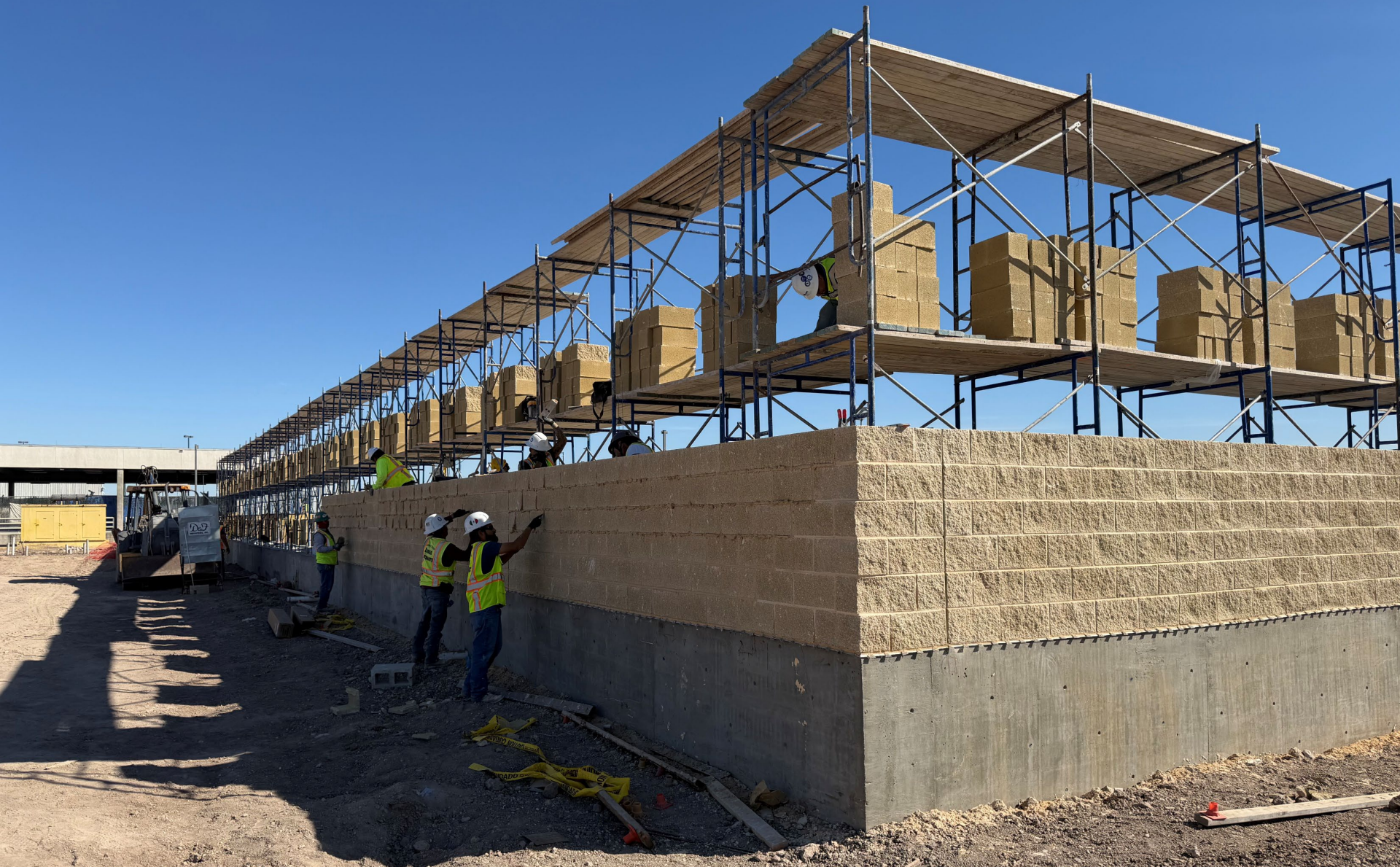
02-05-2026 – the contractor continued scaffolding activities at the Ag Lab. In addition, the contractor began installing 8-inch CMU block along the west and north walls of the Ag Lab.
