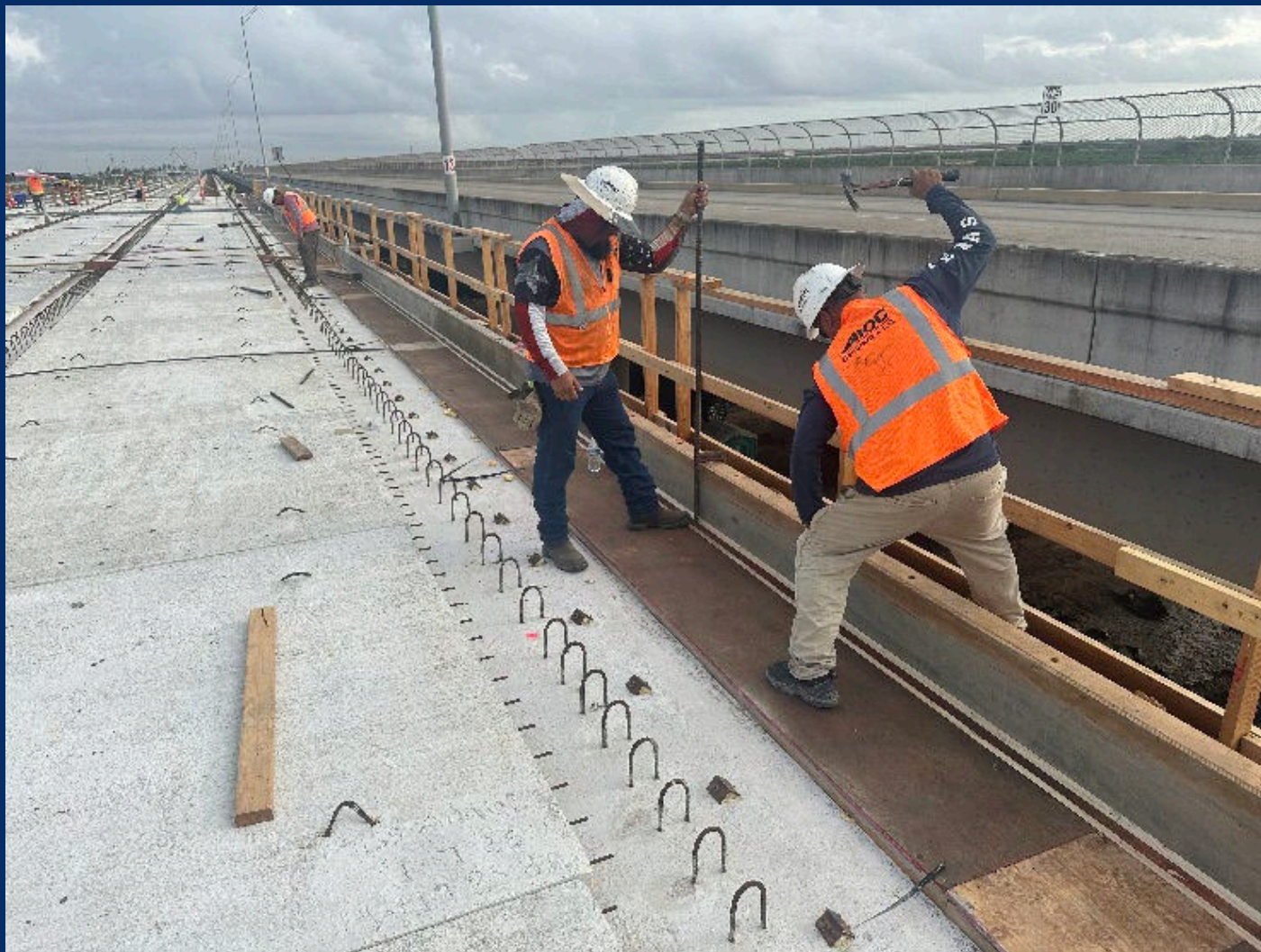
10-14-2025 – Crew installing wood form railings at the east and west ends of Unit 42.
