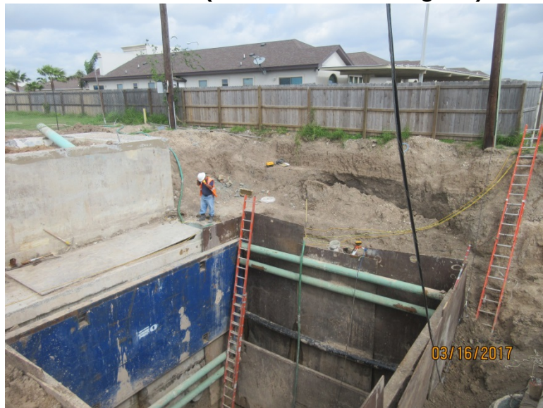
Lift Station #25 and Force Main
