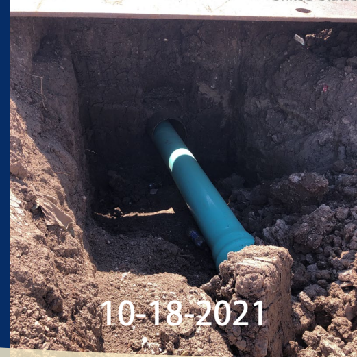
Lift Station No. 30 (1/1)
