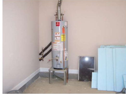
T and P discharge to the floor
