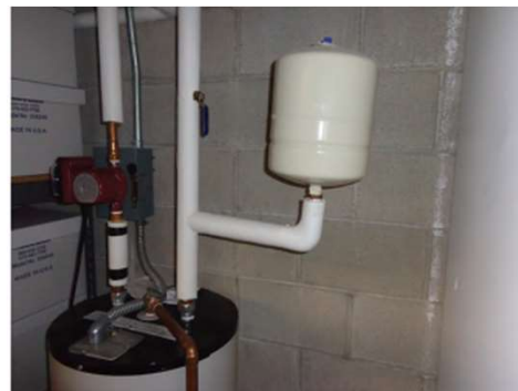
Unsupported thermal expansion tank
