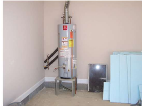
T and P discharge to the floor
